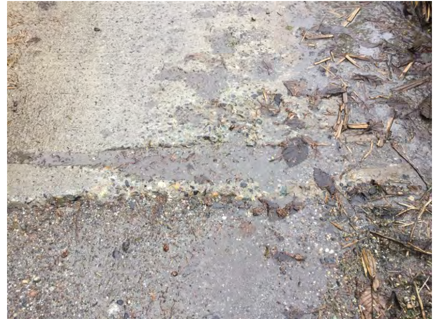
Some deck damage - no rebar noted
