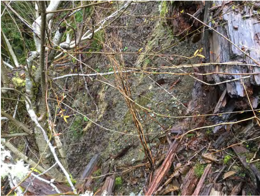
Fill on right downstream banking eroding
